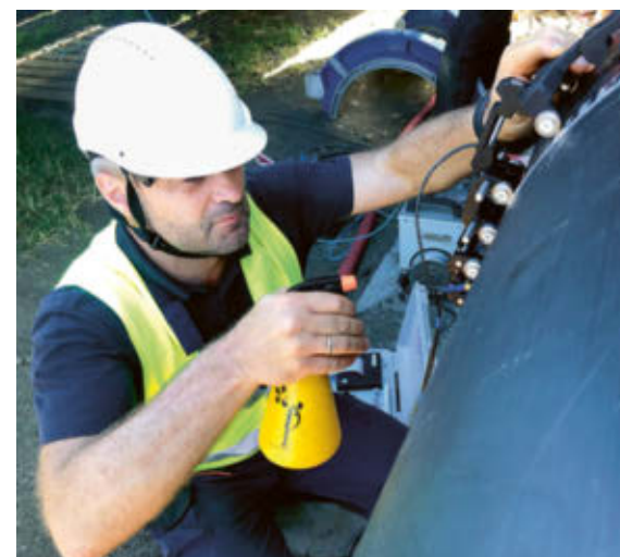
↑ Inspectors in Tahiti use scanners to check the weld beads on pipes. The scanners needed to be prepared for this task.
