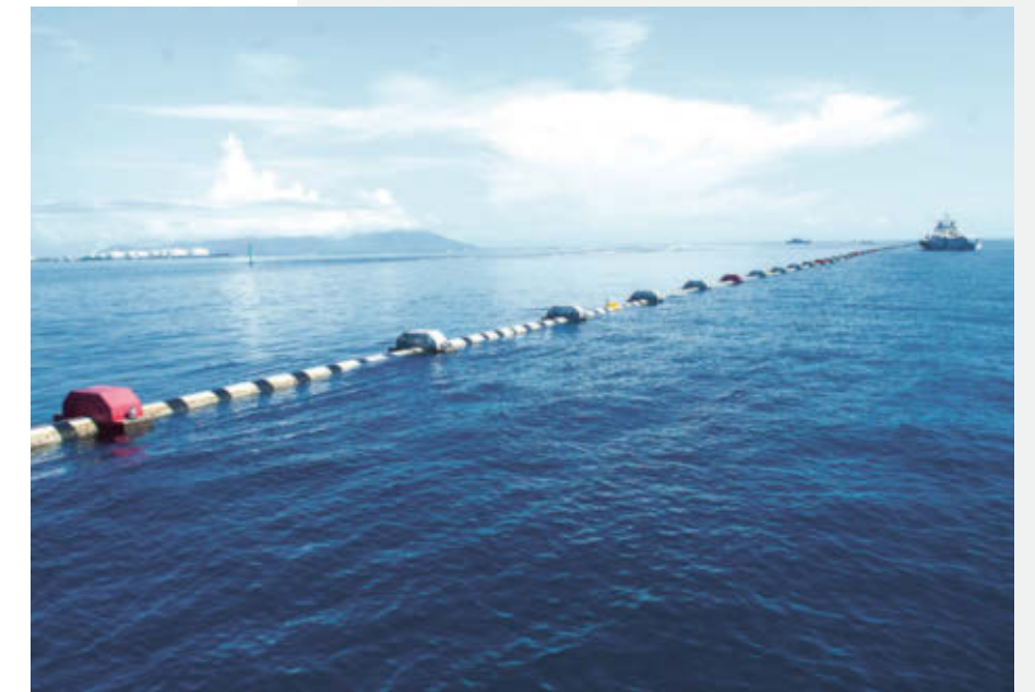
↑ A pipe measuring nearly 4 kilometers in length cools the capital’s new hospital using seawater.
